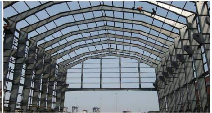
Indian Railway Gantry Building W - Clear Span 20m L - 60m H - 16m
